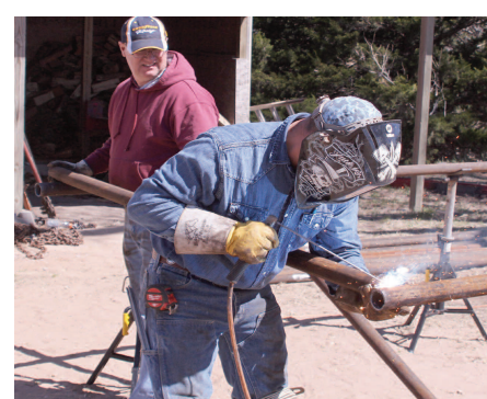
With some help from Chris Ragan, welder Kevin Riffey puts together a metal corner for a pasture fence. Grassland manager Ted Alexander had 7,000 acres of grass and needed 150 new corners to get his pasture fences back in operation. The welders were putting out a corner section every 12 minutes. All the pasture around Alexander's home place was burned but none of the buildings or equipment was damaged. Photo by Gale Rose
