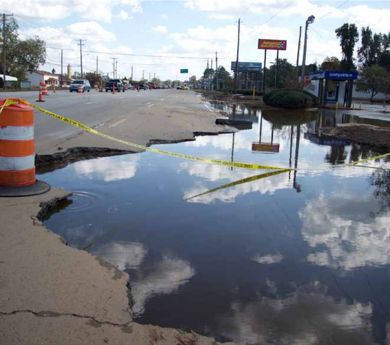
A large portion of US-70 East collapsed due to flood water between Piggly Wiggly and King's Restaurant. The major thoroughfare reopened with one lane traveling in each direction Tuesday afternoon. Photo by Zach Frailey / The Free Press
