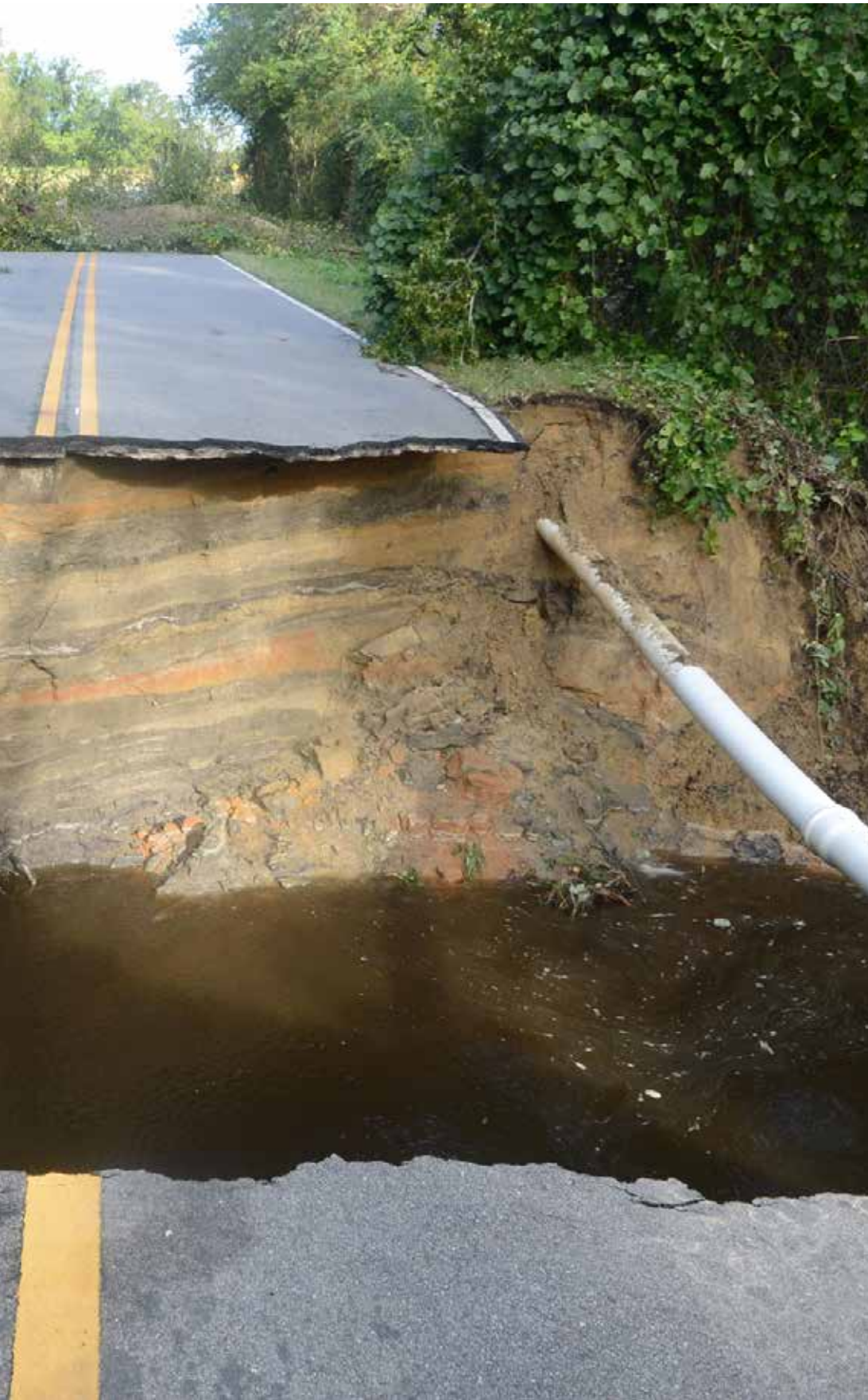
Falling Creek Road is un-passable after rains from Hurricane Matthew caused a portion of the road to collapse. Photo by Janet S. Carter / The Free Press
