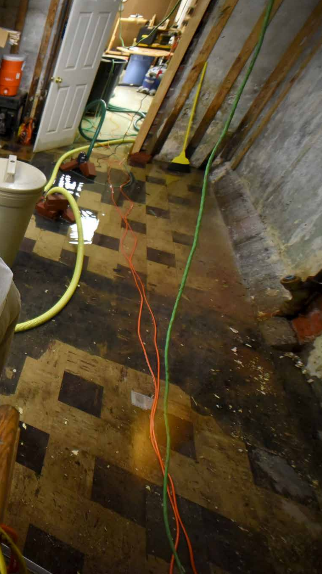
Hardy Creech, owner of Realo Discount Drugs, monitors multiple sump pumps in the basement of his business at 300 N. Queen St. as water from the flooded Neuse River flows into downtown Kinston Thursday evening. Paul Stephen/GateHouse Media
